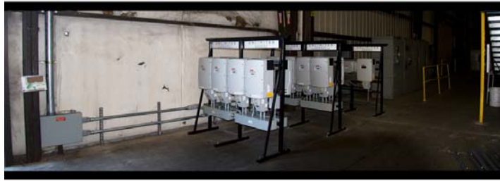
EVAPCO WEST 100KW SYSTEM 17 SMA 6000 us
