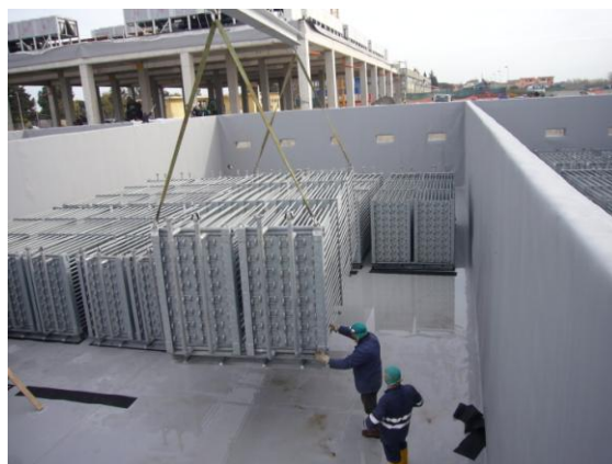
EVAPCO Thermal Ice Storage Installation
